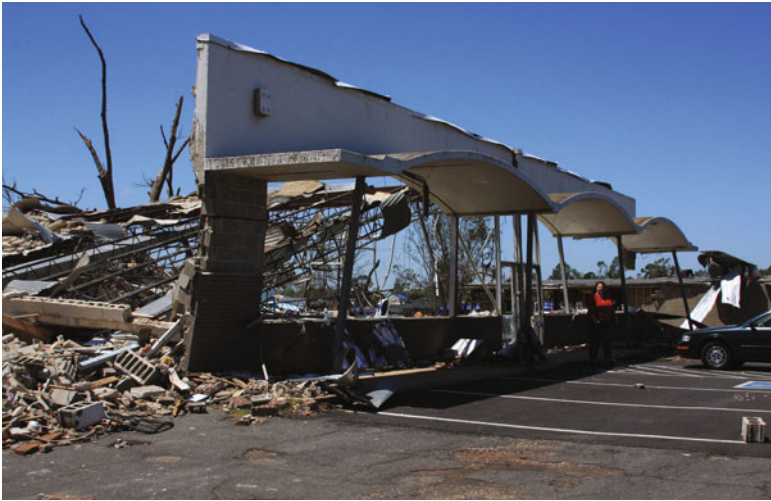
Commercial damage in Tuscaloosa, Alabama, from the April 27, 2011 tornado outbreak. Nearly 11,000 buildings were damaged in the EF-4 Tuscaloosa–Birmingham tornado.
