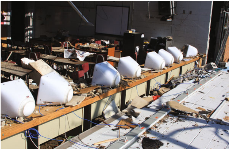
Damage to Joplin High School, Joplin, Missouri, which was destroyed by the May 22, 2011 tornado.
