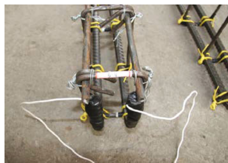
Fig. 9 Pre-wired cable of the bar
