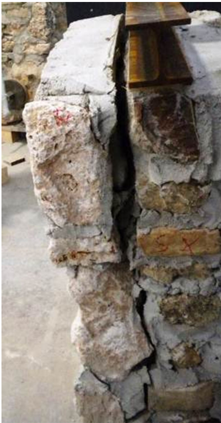
Fig. 7 Failure mode (unreinforced panel)
