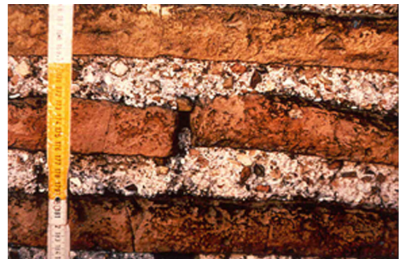
Fig. 13 View of thick mortar joints of St. Vitale basilica in Ravenna (Italy)
