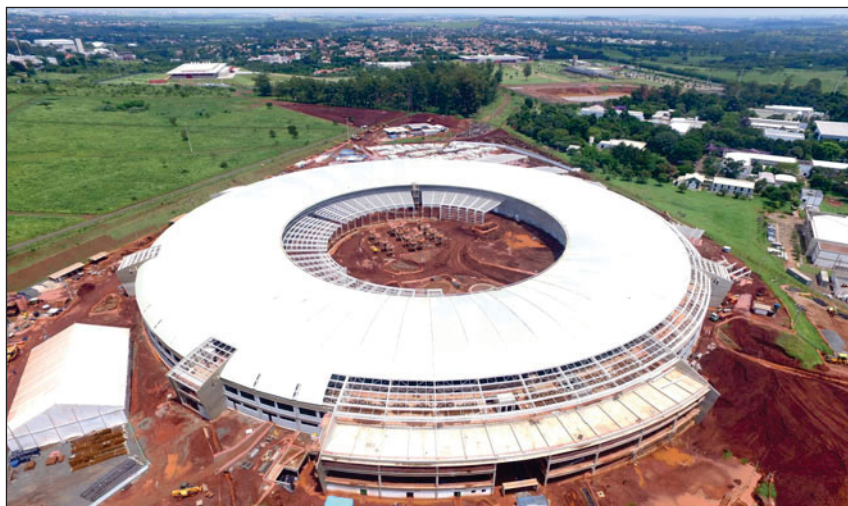
The construction site of Sirius, Brazil's new fourth-generation synchrotron light source. Sirius could greatly increase the capacity of Brazil's research infrastructure, but scientists are already struggling to maintain adequate support for existing research. Credit: LNLS/CNPEM.
