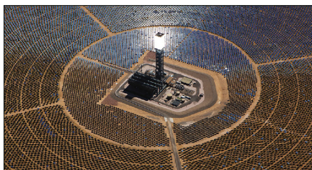
Mirror assemblies that focus the power of the sun on solar receivers atop power towers at the Ivanpah Solar Electric Generating System in California’s Mojave Desert. Credit: BrightSource Energy.
