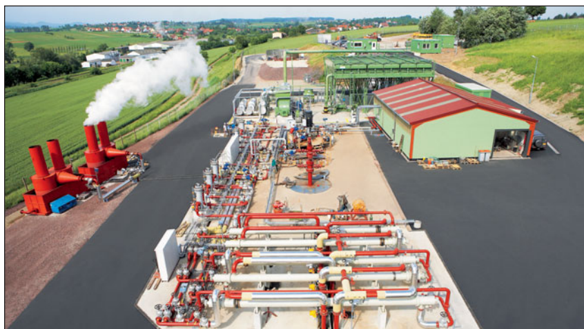
The European Geothermal Hot-Dry-Rock Project enhanced geothermal systems plant in Soultz-sous-Forêts, France, produces thermal energy from fractured crystalline rock for electricity. It also serves as a platform for basic research and testing. Photo courtesy of Groupeement Européen d'Intérêt Economique "Exploitation Minière de la Chaleur" (GEIE EMC).
