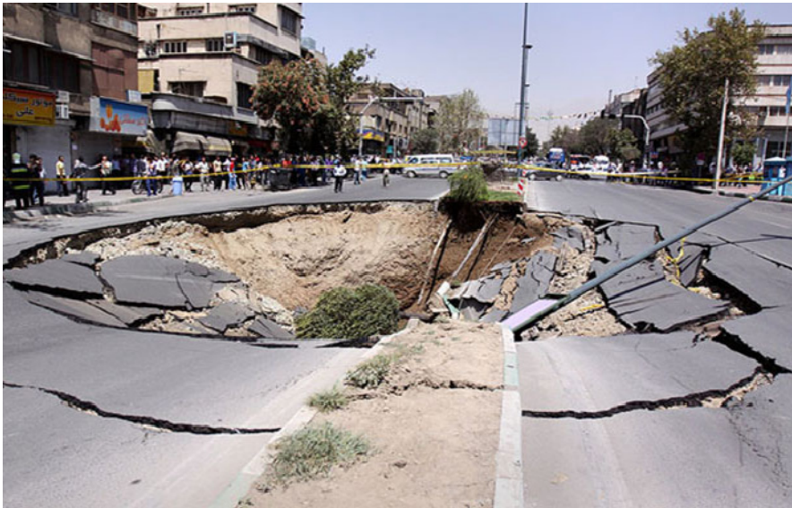
Fig. 1. Surface settlement of Navab Str., Tehran, Iran, due to an obsolete Qanat tunnel collapse (Donya-e eqtesad 2009).
