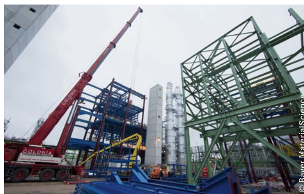
The foundations have been laid ready for the building of the steel structure. Completion and start of operation of the new high-tech plant for the production of the chemical TDI (toluene diisocyanate) are planned for mid-2014.
