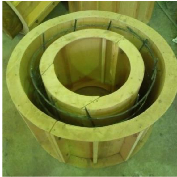
Fig. 4 A wooden mold of pipes
