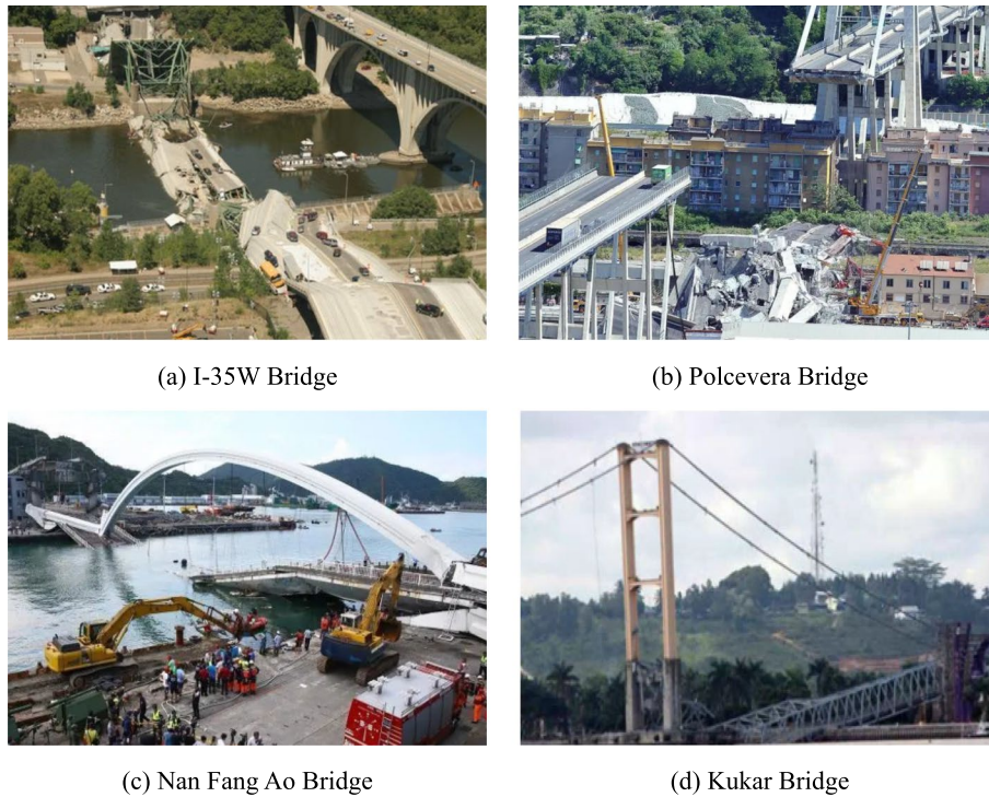
Fig. 1 Accidents of large span bridges
