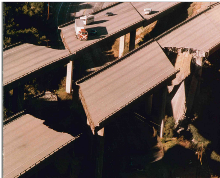
Fig. 1 Unseating of Gavin Canyon Bridge in the 1994 Northridge Earthquake
