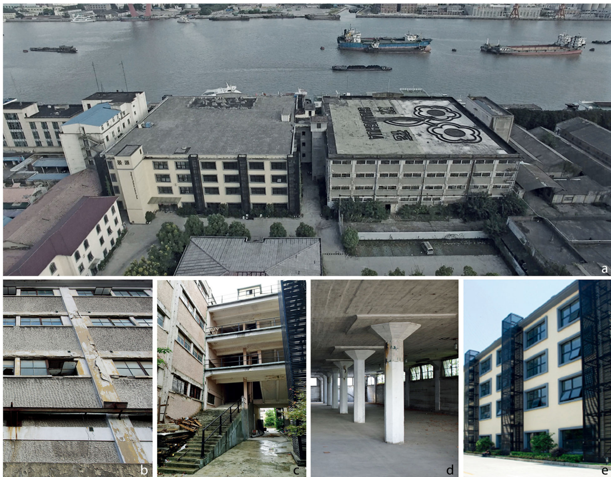
Fig. 6 Yong'an Warehouse before the renovation. a: aerial view of the site. b: destroyed exterior walls. c: the connection between the east and west wings. d: interior space. e: renovated eastern warehouse: office building (Source: Archi-Union Architects)
