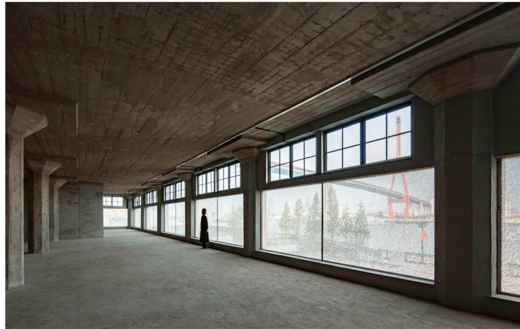
Fig. 8 Renovated beam and slab structures on the top level (Source: Tianzhou Yang)
