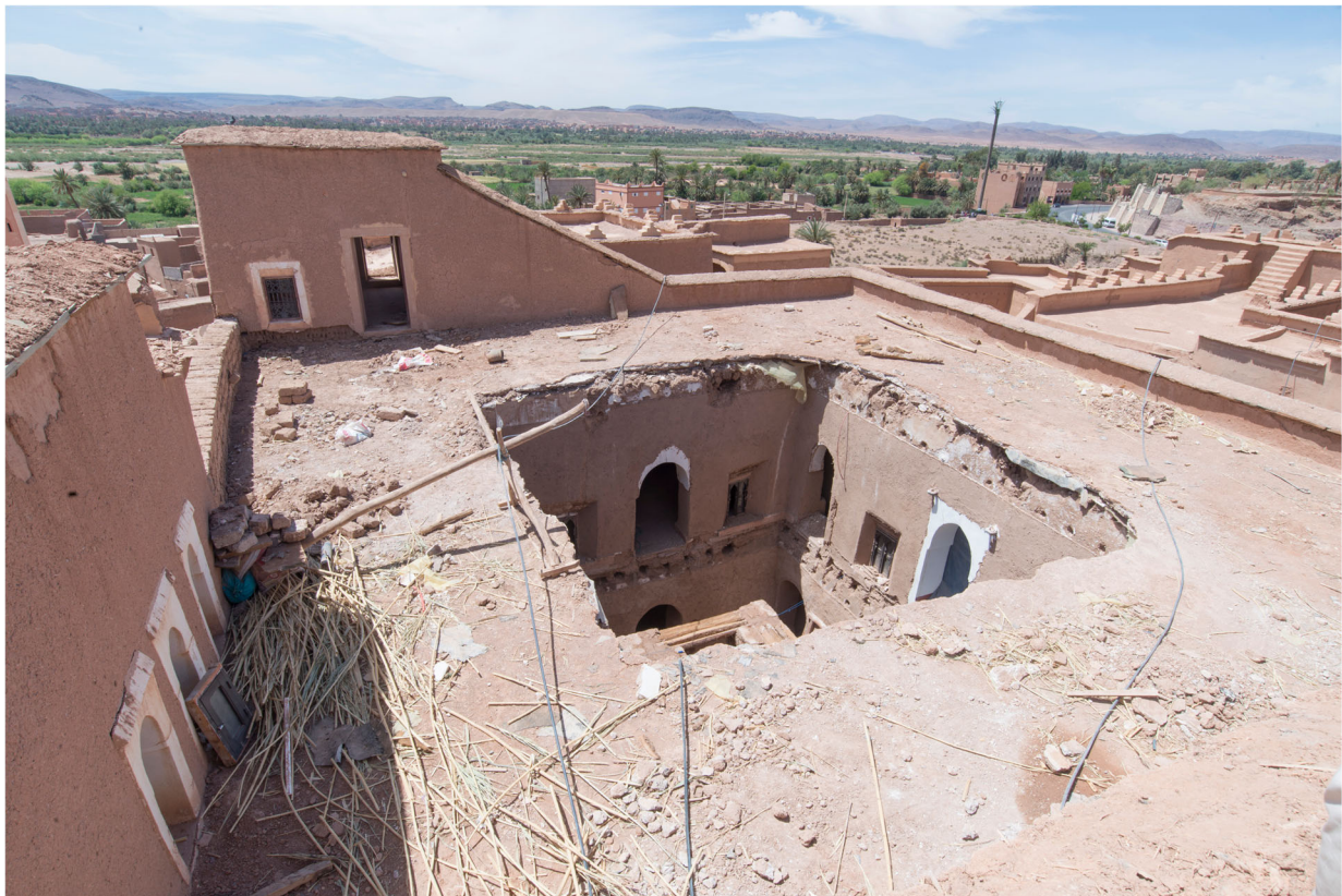
Fig. 3 Damage to earthen architecture structures from strong rains, Ouarzazate, Morocco (2016) (Source: the authors)
