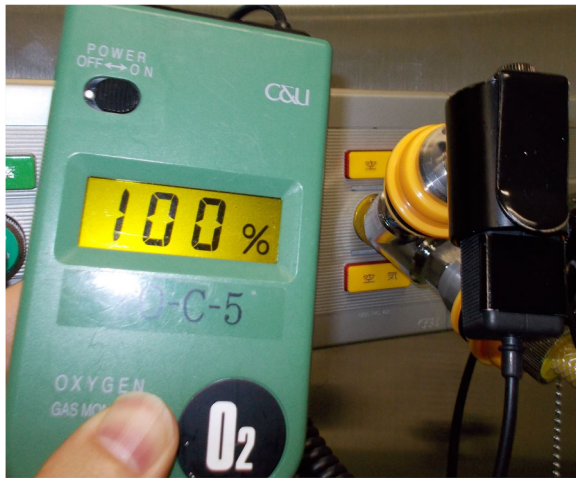
Fig. 1 Oxygen-rich air of up to 100% oxygen was occasionally detected by a handheld oximeter (XO326-BC, New Cosmos Electric, Osaka, Japan) connected to medical air outlets in certain operating rooms
