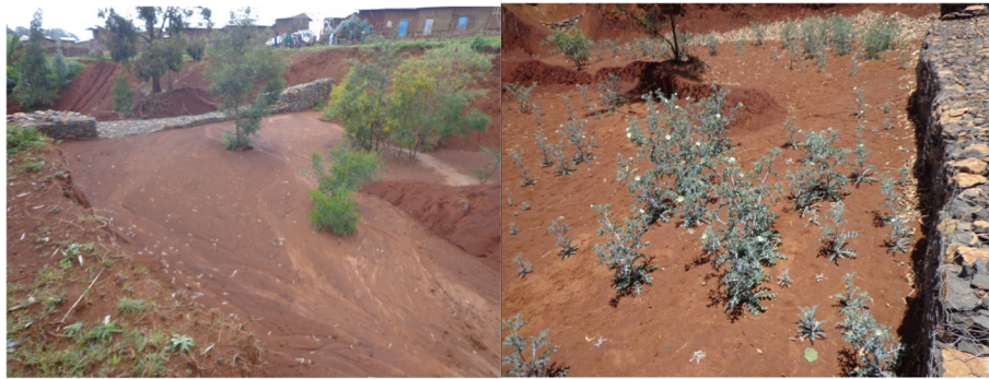
Fig. 2 Example SSD pictures constructed to sequester sediment and SOC two years old (left, Segno Gebeya watershed) and five years old (right, Woybila watershed), in the northwest highlands of Ethiopia
