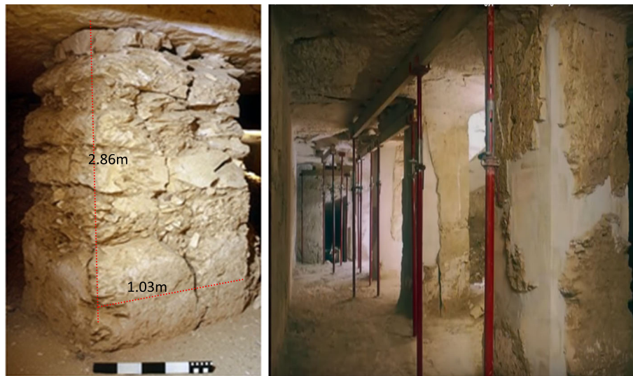
Fig. 35 Present state of the sixteen supporting rock pillars in the Chamber 3. which are structurally damaged. Vertical cracks due to the overloading and strength regression are obvious ( http://www.thebanmappingproject.com/ ). Permission was granted by Weeks, K.R. © Theban Mapping Project 2006 to reuse this figure
