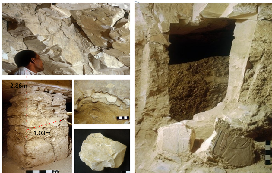
Fig. 8 Extensive structural damage in KV5. Engineering failure of the structural pillars, sidewalls and Ceiling of the Corridors and Chambers in the KV5 ( http://www.thebanmappingproject.com/ ). Permission was granted by Weeks, K.R. © Theban Mapping Project 2006 to reuse this figure
