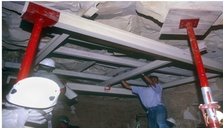
Fig. 29 Temporarily support system for the KV5, installed recently by the Theban Mapping Project. After TMP. Permission was granted by Weeks, K.R. © Theban Mapping Project 2006 to reuse this figure.
