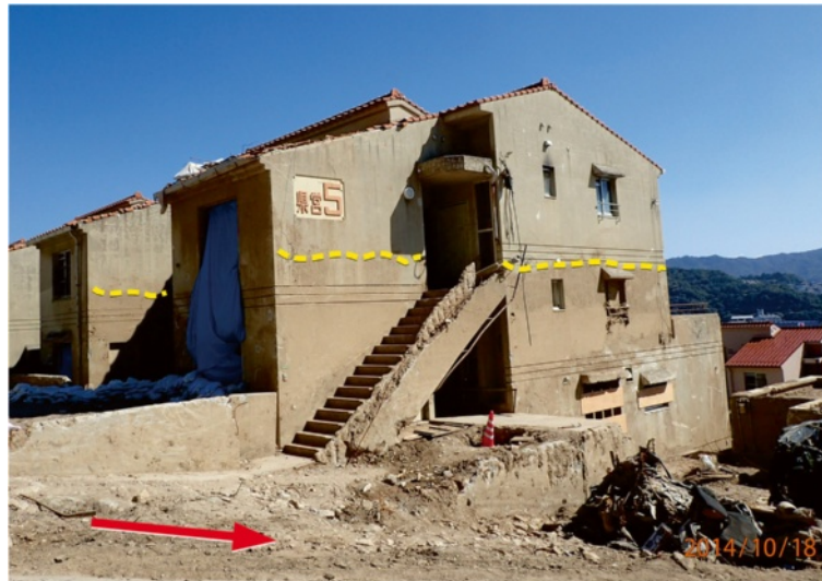
Fig. 8 The damaged prefabricated housing at the pathway of the Midori-ga-oka debris flow. From the muddy trace on the wall, the flow depth of debris flow was about two-floors high
