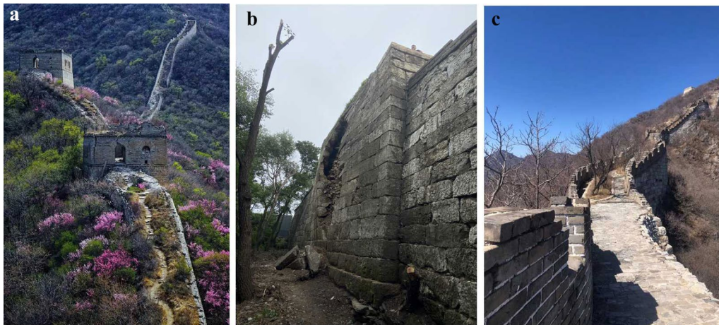
Fig. 2 The Dazhuangke Great Wall. a Before protective repairs; b Deterioration of the Dazhuangke Great Wall; c After protective repairs
