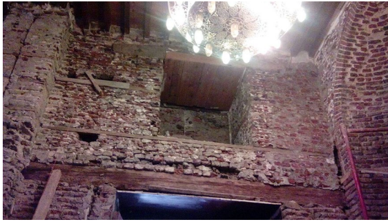
Fig. 19 Extensive disintegration and degradation of the bricks walls of the church due to the subsurface water rising
