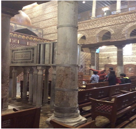
Fig. 23 Strengthening and reinforcing of structural marble and granite columns with steel ring beams
