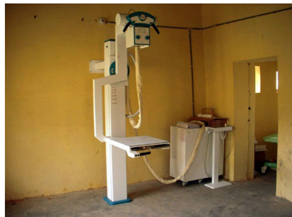
Figure 2 Nyaya Health X-Ray Installation. Note the protective screen around the control room had yet to be installed in this photograph.
