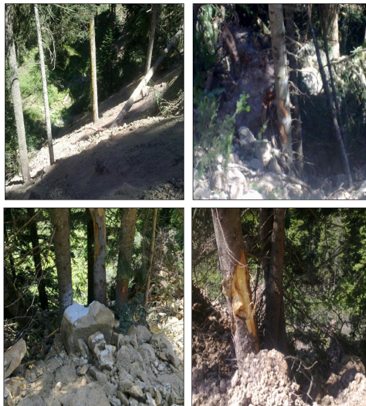
Figure 4 Tree damages during forest road construction.
