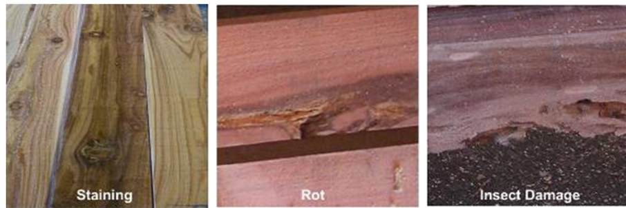
Figure 7 Examples of staining, rot and insect damage observed in redwood boards during timber grading.
