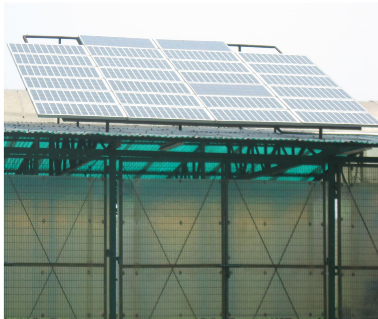
Fig. 3 A solar charging station at CSIR-CMERI, Durgapur
