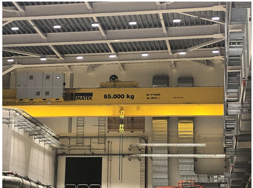
Fig. 207 Largest existing ESS overhead crane currently in operation in the D02 Target building
