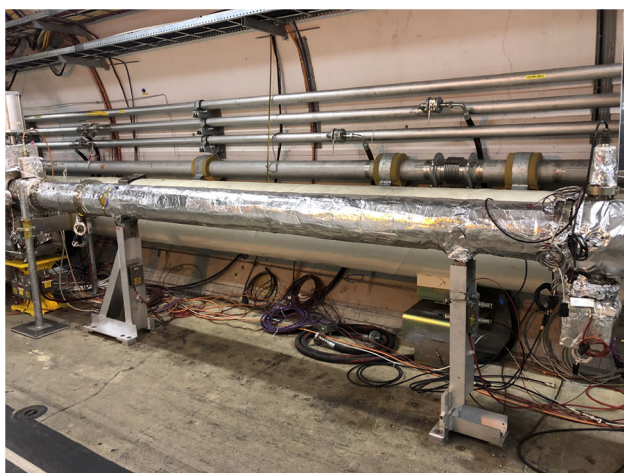
Fig. 3 Conditions inside the LHC tunnel at the proposed location. Good accessibility and space availability allow for easy installation of the crystal assembly
