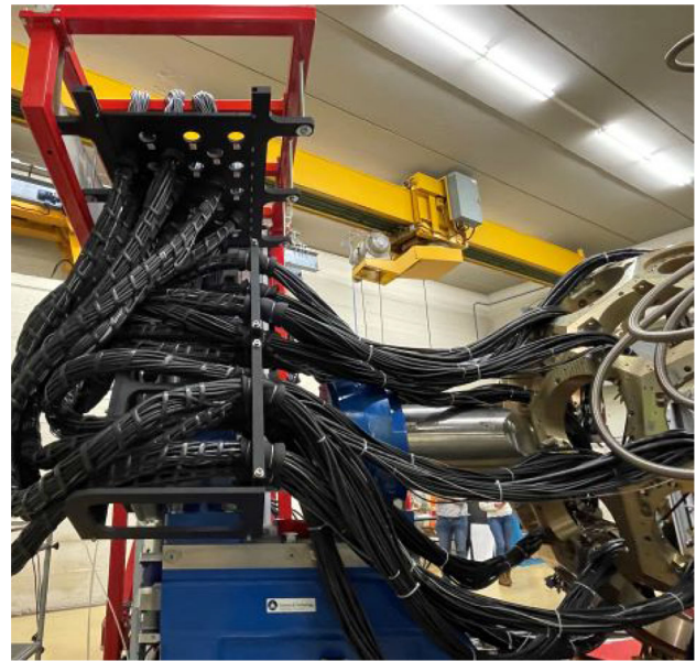
Fig. 21 Cable management system allowing for the array movements (rotation and translation)
