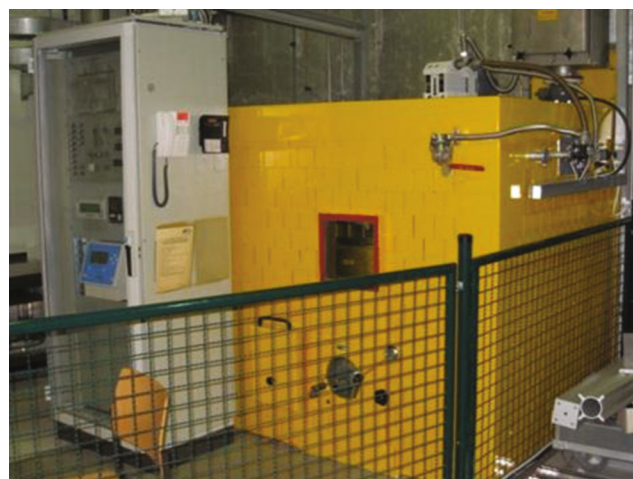
Fig. 24. General view of the pneumatic transport system and control rack (prototype).
