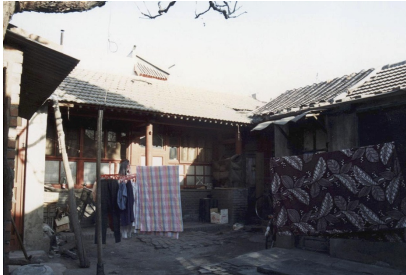
Figure 5. Deteriorated courtyard housing in Beijing.
