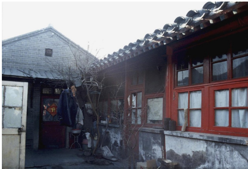
Figure 6. Deteriorated courtyard housing in Beijing.
