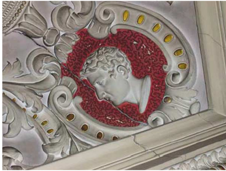
Figure 3: Cracking in ornaments (Marquis of Tomar Palace in Lisbon)
