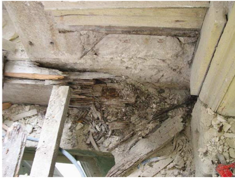
Figure 8: Rot of timber beam next to outer wall, visible only after the pavement was dismantled (Morais Villa in Ponte de Lima, Portugal)
