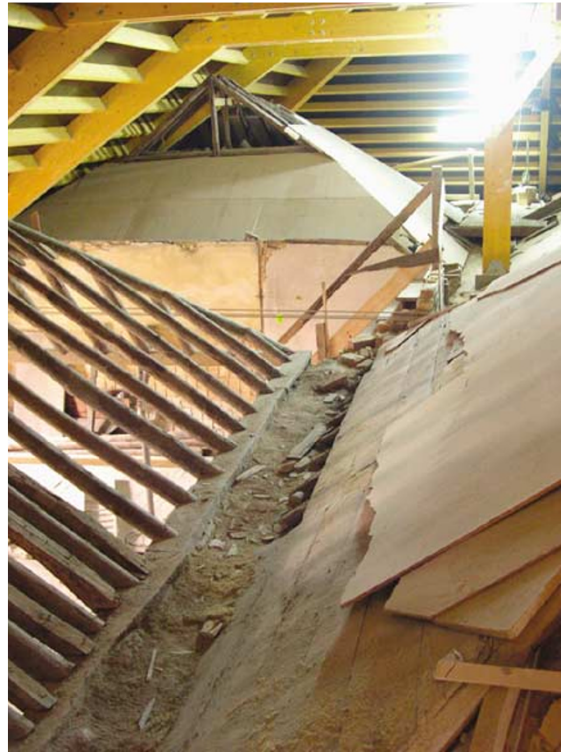
Figure 9: Extrados of plastered roofs: original structure and new support of the roofs (Marquis of Pombal Palace in Lisbon)
