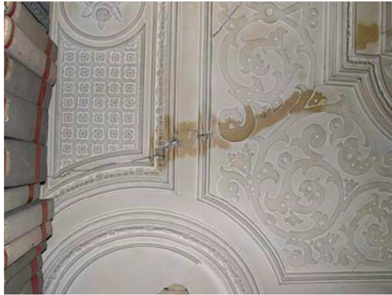
Figure 4: Stains caused by water entrance (Marquis of Tomar Palace in Lisbon)
