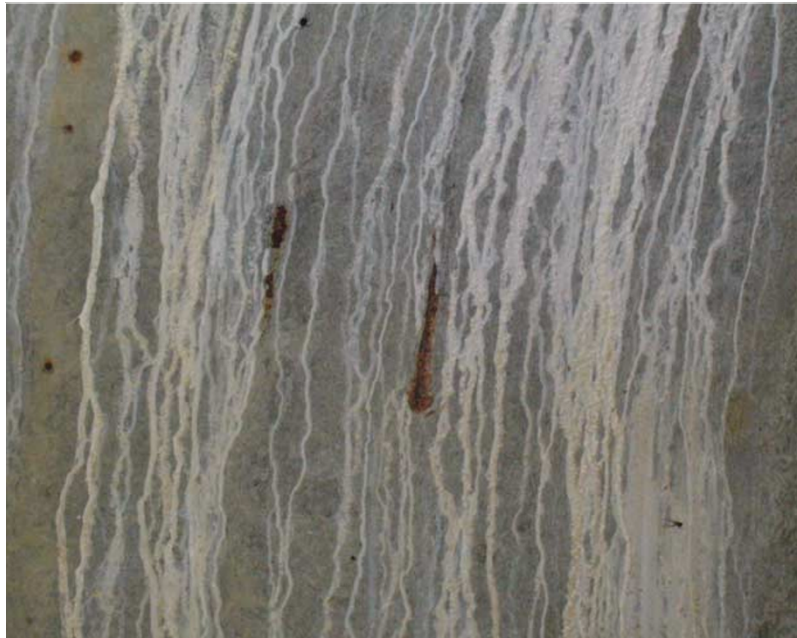
Figure 2: Calcite in cracks and visible corroded rebars
