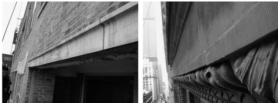
Figure 11: Vertical displacements of terra-cotta units over window openings
