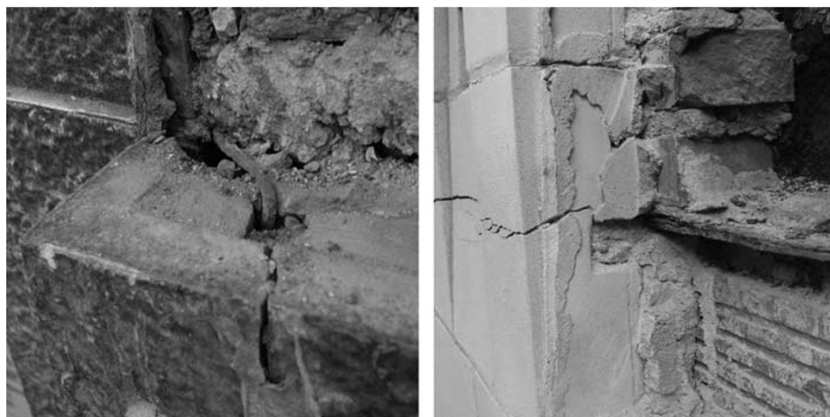
Figure 5: Representative distress of terra-cotta cladding. Cracking at lateral tie (left) and cracking at shelf angle location (right)
