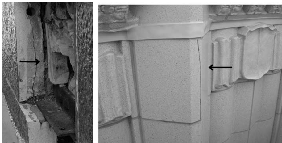
Figure 7: Vertical cracking within the plane of terra-cotta (left) and through the face (right)
