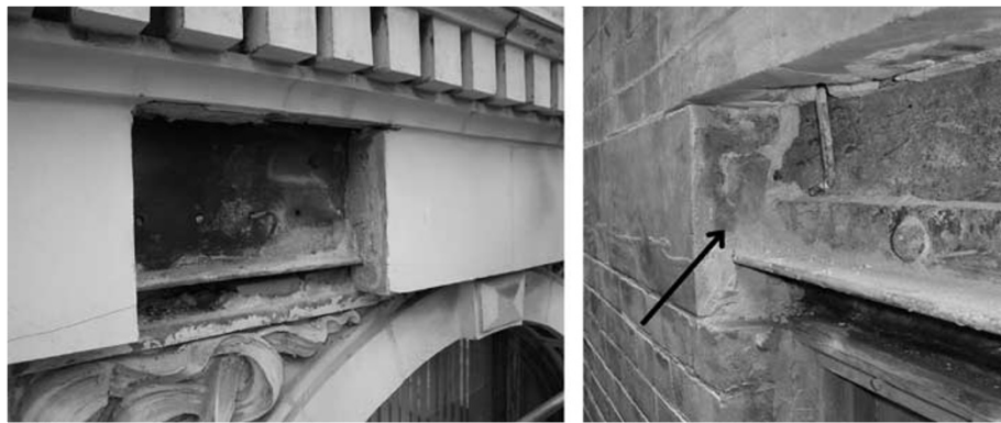
Figure 6: Horizontal cracking at shelf angle locations
