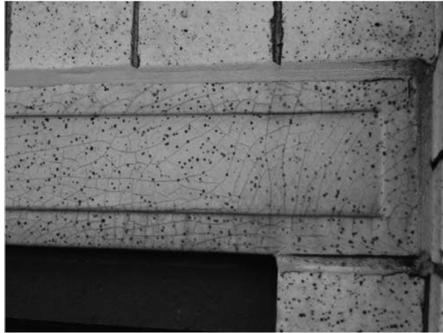
Figure 9: Fine cracks (crazing) reflecting stresses within terra-cotta unit
