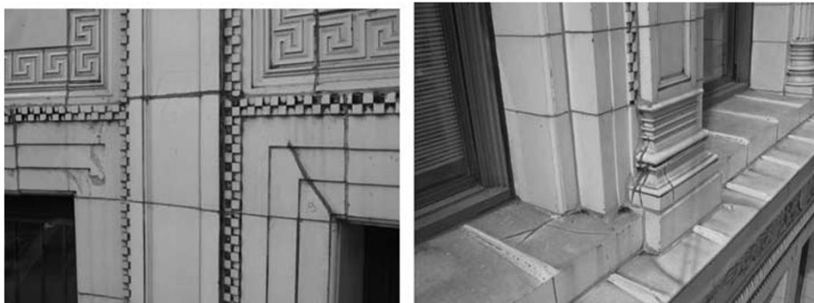
Figure 8: Example of diagonal cracking in terra-cotta
