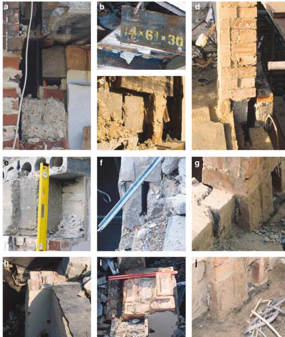
Figure 2: A selection of photographs taken during the deconstruction of the building showing the steels (and dimensions) (b), the support for pier A2 (c), (d), (f), (g) and (j), brick pier dimensions (h) and (i) and a steel-encased beam at B1/B2 (e)
