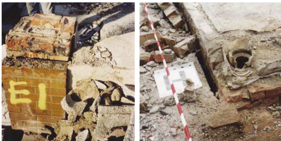
Figure 5: The base of pier E and the detail of the floor slab with gully below
