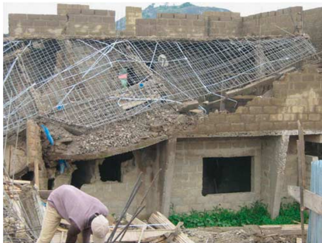
Figure 3: Structural failure: As a result of substandard materials used.
