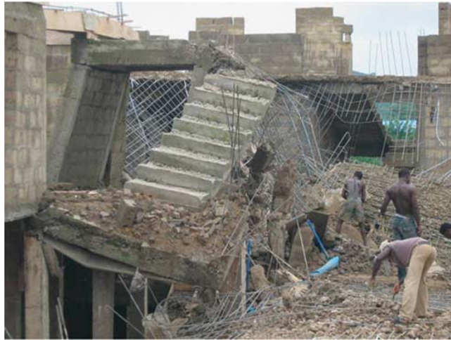
Figure 2: The hotel under construction that collapsed along Oba-Ile road, Akure, showing the wreckage.
