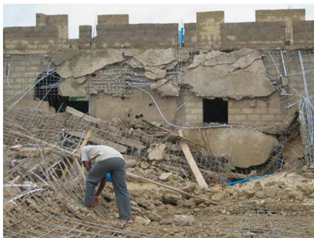
Figure 4: Another view of the collapsed hotel building.
