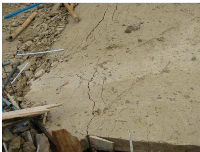
Figure 1: Concrete slab full of cracks and disintegrating from steel reinforcement.
