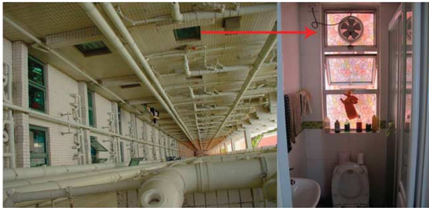
Figure 4: Toilet windows usually face the re-entrant, where the bacteria easily spread through stack effect. Source: Photograph by the authors.
