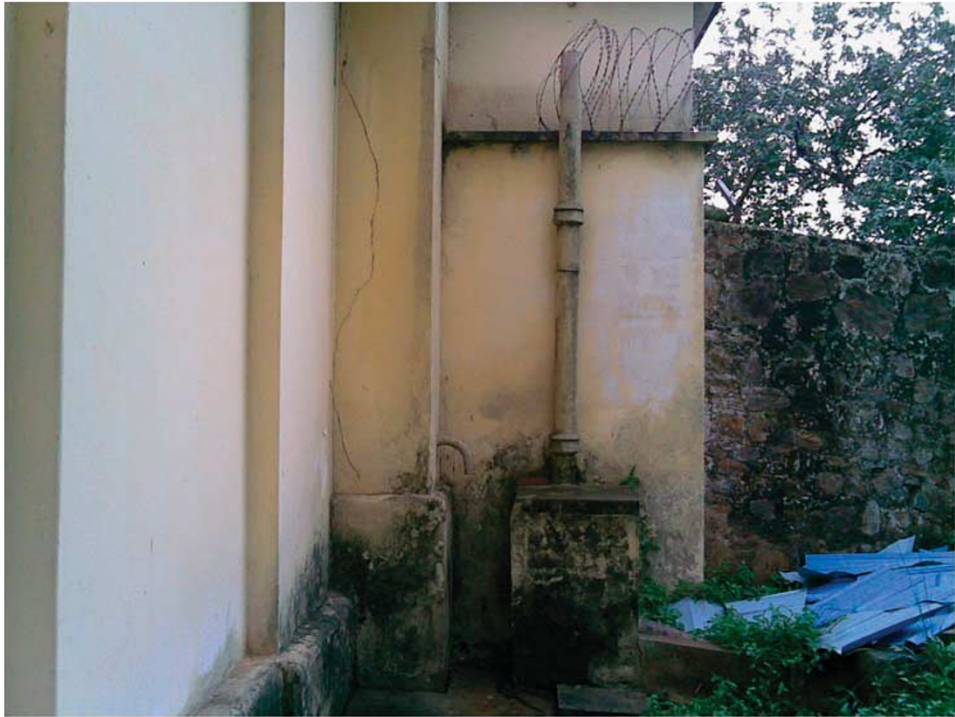
Figure 2: Deterioration – Cracks and moss growth on National Museum wall.
