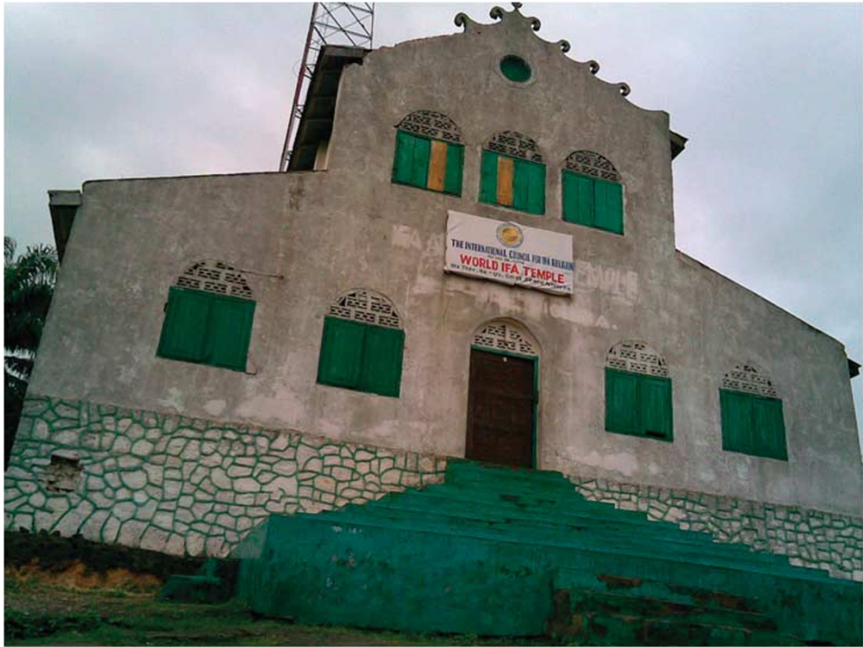
Figure 3: World Ifa temple – Deteriorating external works.
