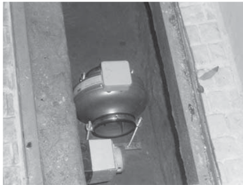
Figure 14: Electric equipment to force ventilation.
