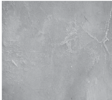
Figure 4: Efflorescences in the rendering cracks.
