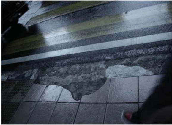
Figure 3: A damaged paving at Tun Perak street. Note: These broken paving and damaged floor show that quality of paving is improper in Tun Perak street.
