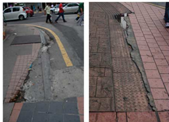
Figure 2: Different parts of Bukit Bintang street paving. Note: These broken paving and damaged floor show that quality of paving is improper in Bukit Bintang Street.
