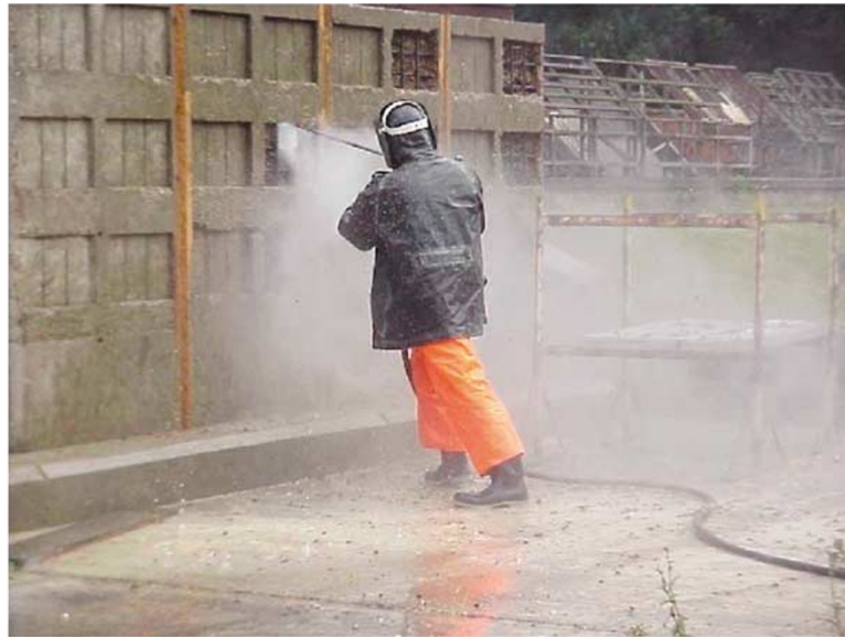
Figure 2: High pressure water jetting to remove damage concrete and prepare for repairs
