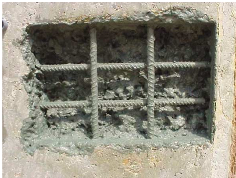
Figure 3: After removal of damaged concrete; the reinforcement is treated before repairs are made with concrete or a proprietary material
