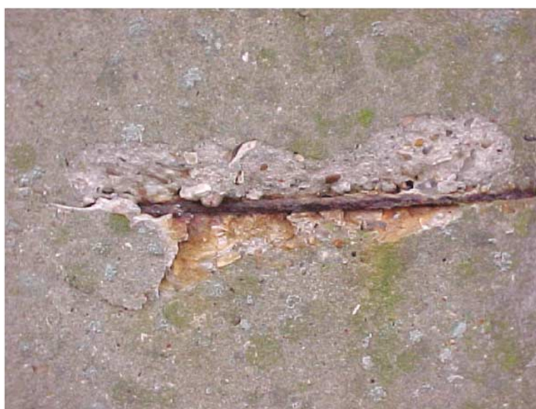
Figure 1: Corroding reinforcement causes concrete to crack and spall
