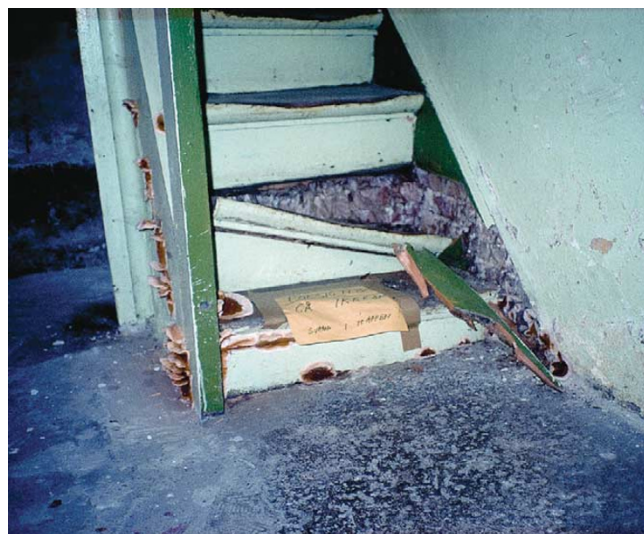
Figure 7: Fruiting bodies of the dry rot Serpula lacrymans breaking out on a totally decayed staircase in a cellar
