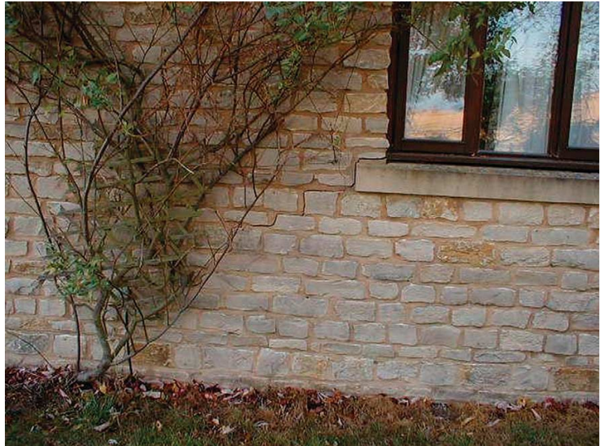
Figure 5: Cracking in a recently built house near Stratford-upon-Avon. This house is less than five years' old and the design of the foundations did not account for poplars, willows and maples growing in the garden at distances of between 10 m and 20 m from the house
