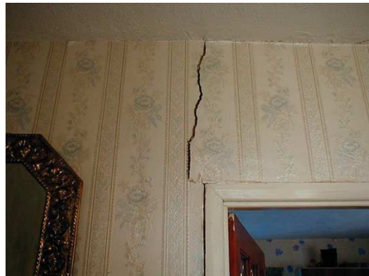
Figure 6: Internal cracking in a farmhouse in Lincolnshire caused by poplar trees 20 m away from the building
