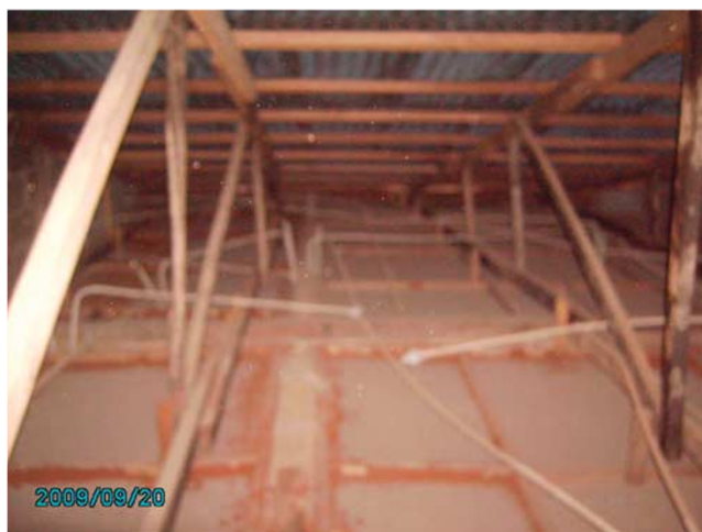
Figure 5: General arrangements of the wooden roof trusses and termite attack on the noggin.
