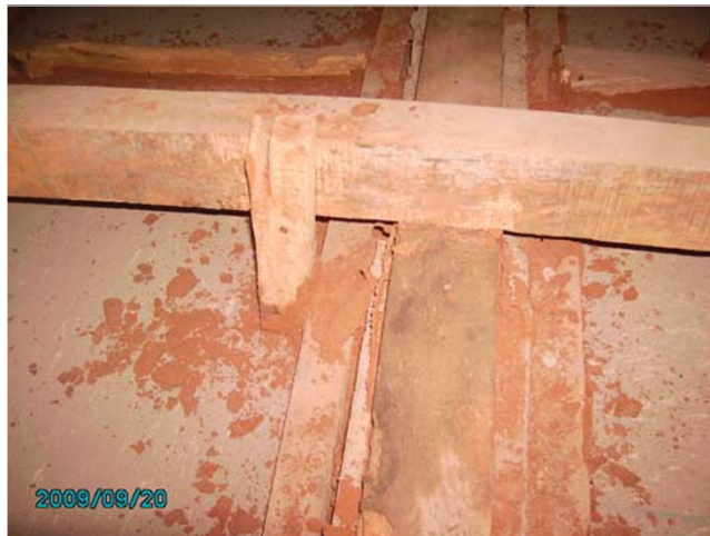
Figure 4: Termite attack on the wooden noggin.
