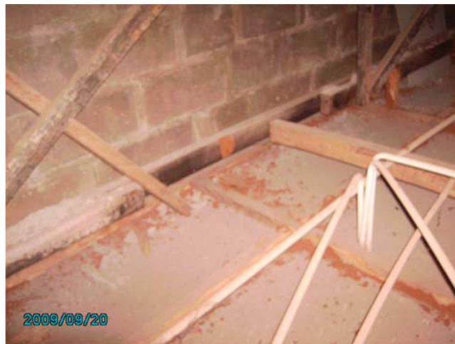
Figure 2: Termite attack on the wooden noggin.
