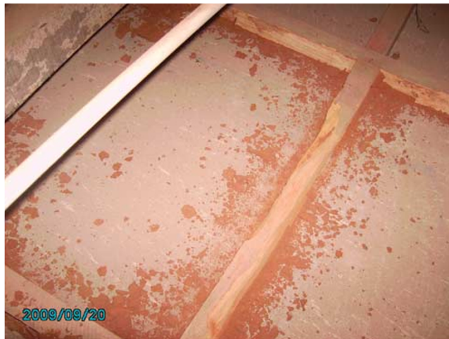
Figure 3: Termite attack on the wooden noggin.
