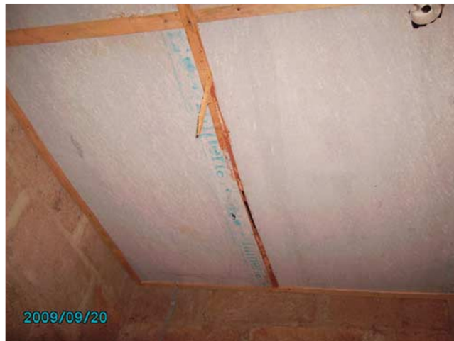
Figure 1: Termite attack on tie-rods connecting the ceiling asbestos to the roofing noggin.
