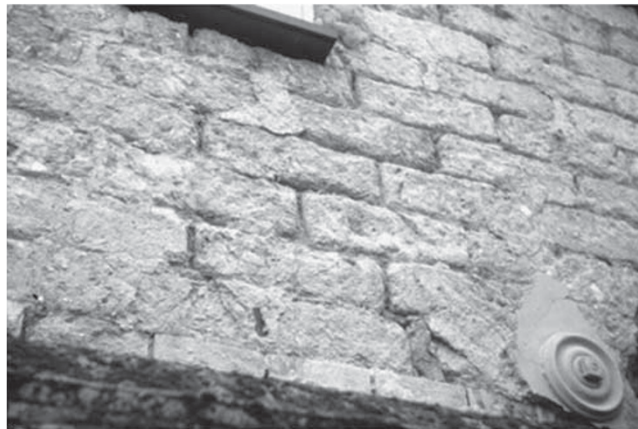
Figure 2: Clay lump exposed for repair in Shipdham, Norfolk.
