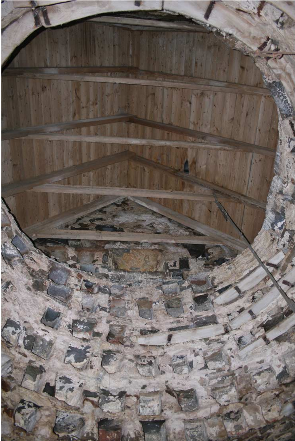
Figure 2: Interior of Auchmacoy Doocot: Note the stone, slate and lime constructed boxes, the high-level timber alighting ledges and the reconstructed timber roof.
