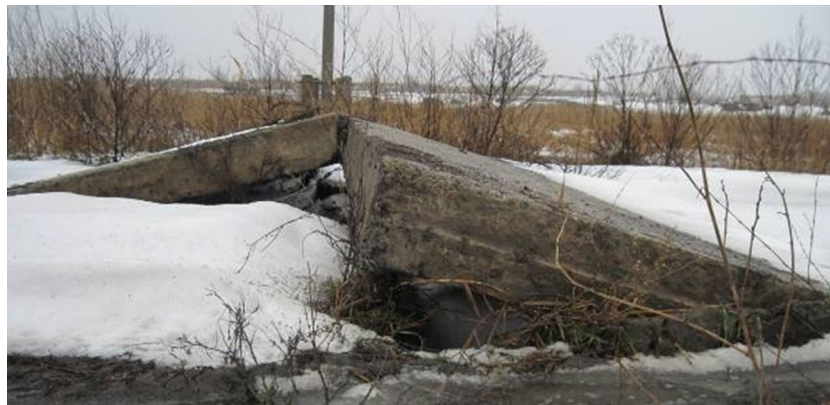
Figure 1. View of the damaged road surface due to the impact of mining operations (automobile road above the underground mine).
