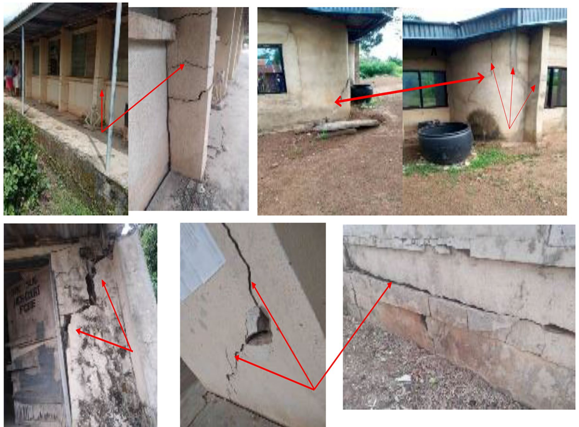
Figure 11. Horizontal, Diagonal and vertical cracks on buildi.
