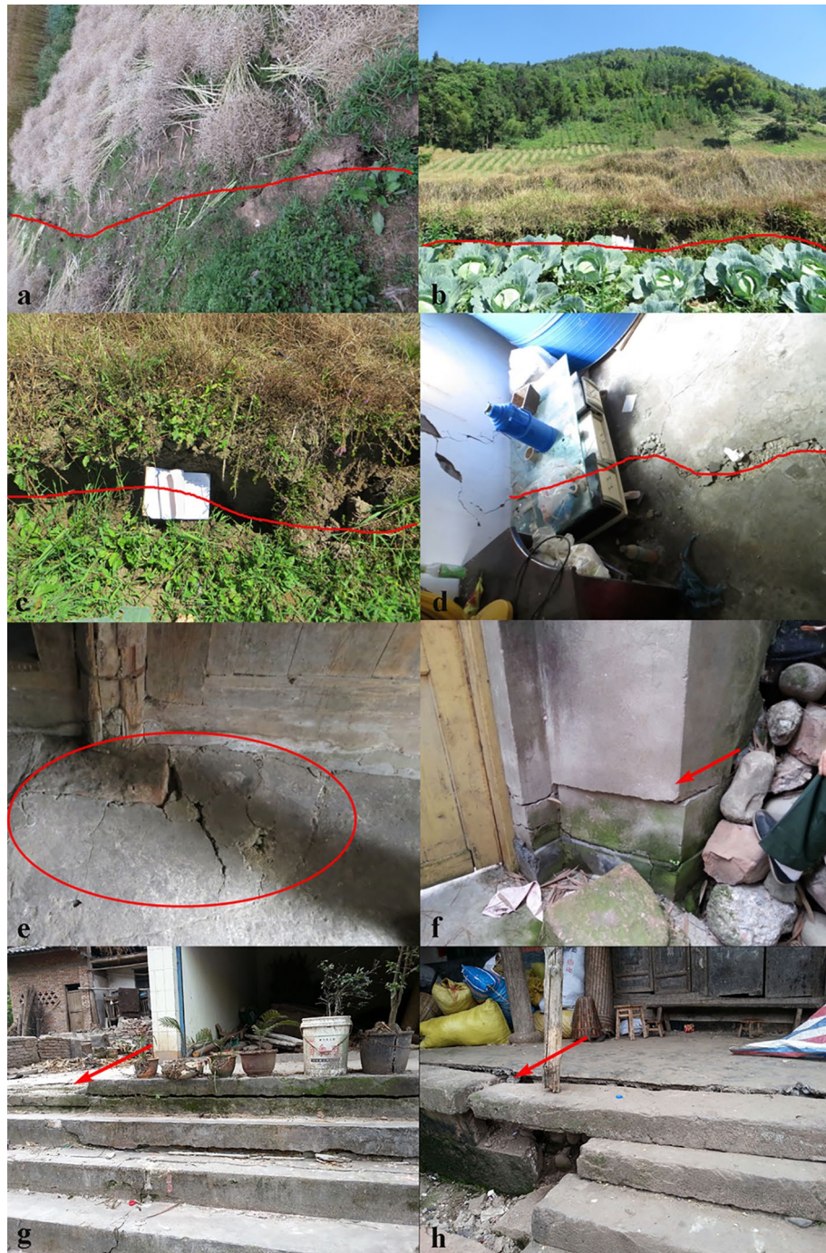
Figure 5. Macroscopic deformations have been observed within the landslides body. (a) Crack C1. (b) Crack C2. (c) Crack C3. (d) Crack C5. The locations of bulges and dislocations are shown in Fig. 4.
