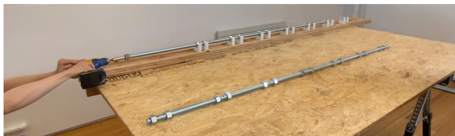
Fig. 17 After all the hex nut locators were properly placed, a threaded rod is screwed through jig
