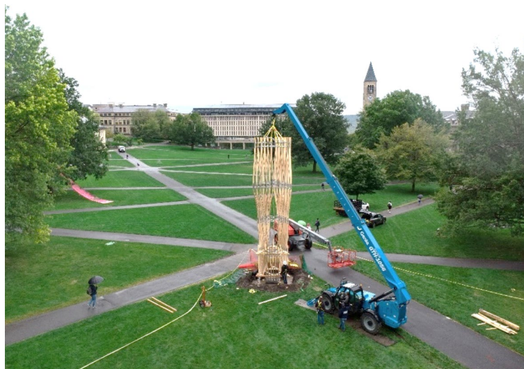
Fig. 22 Aerial photograph of the Unlog Tower lifted on the foundation pad with a boom forklift, photo by Cynthia Kuo
