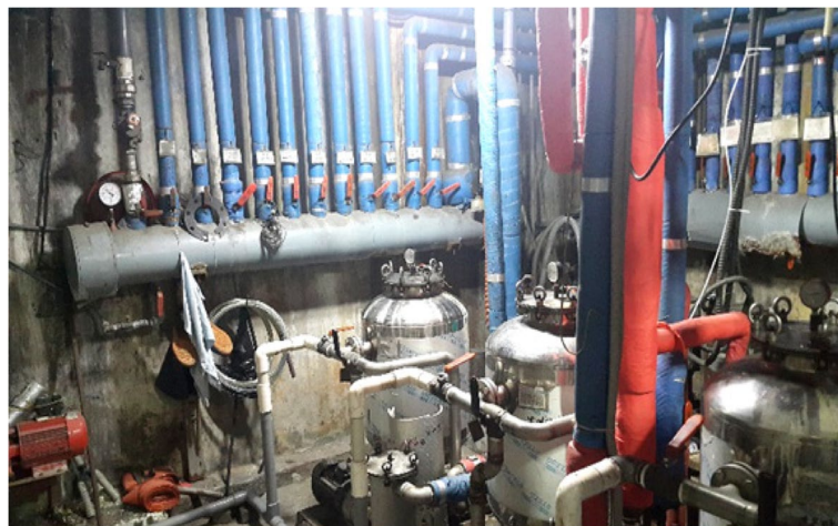
Fig. 3 Sand filter and supply pipes for bathtub water in the basement machine room
