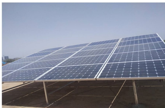
Fig. 3 PV array at the top of the ERC
